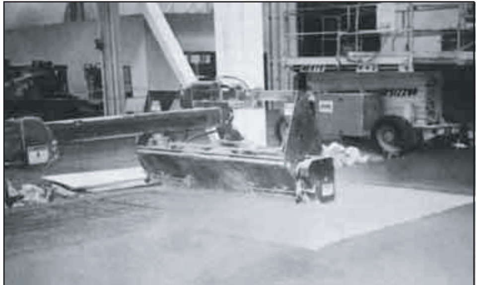
Figure 1. A mechanical spreader applies a metallic dry-shake hardener to the floor surface to improve abrasion resistance.
