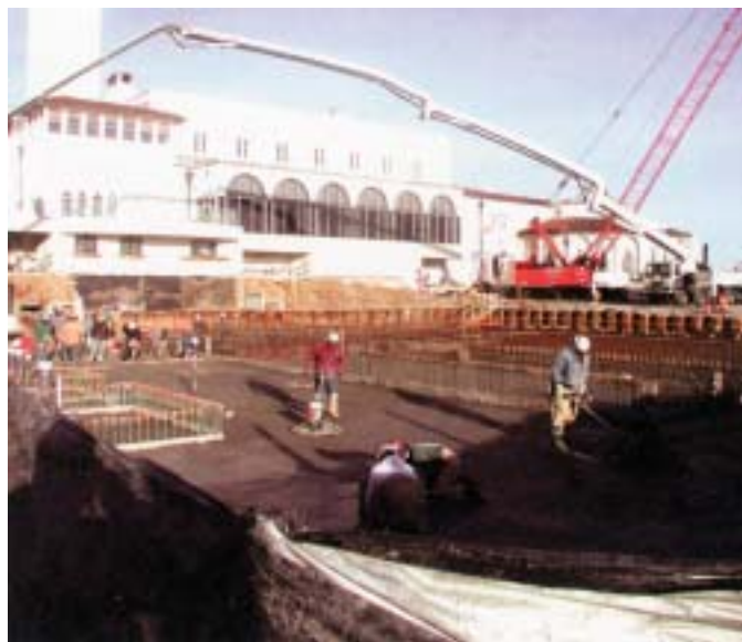
Fig. 2: Placing concrete in February at the Grosse Pointe Yacht Club in Grosse Pointe, MI. Within 2 h of placement, two finishers using machines with float blades were on the concrete. Within 4 h of initial placement, two finishers on kneeboards were putting a hard-troweled finish on the tunnel floor areas that had been previously floated
